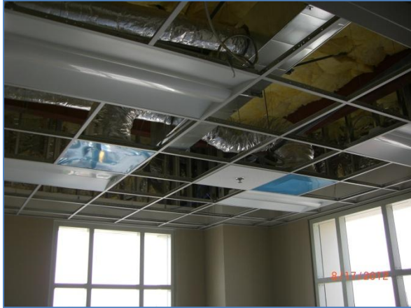
Ceiling grid, light, diffuser, and fire sprinkler
