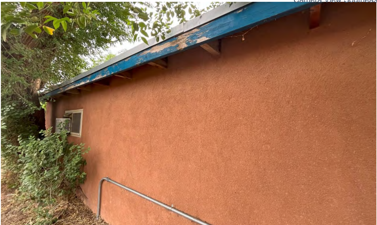
Frame 8. HCPI 54937 Northwest Elevation showing protruding wooden eaves and new stucco and window. Camera View Northeast.
