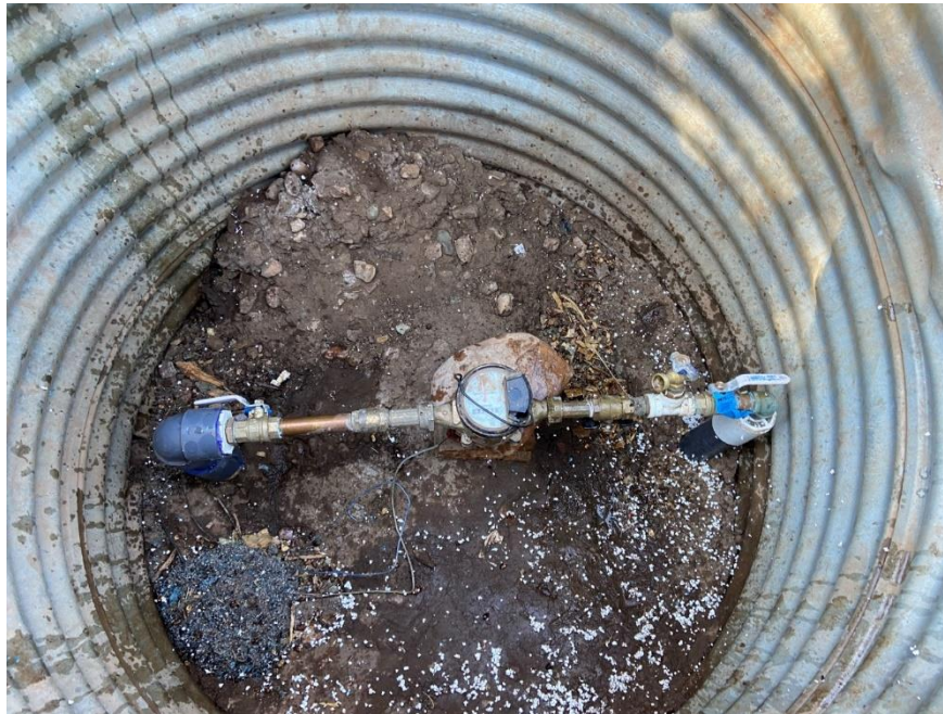
Photo 2 – Redundant 3/4-inch Meter Installed by Hyde Park Estates
