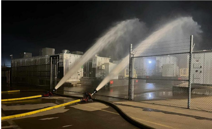
Escondido Substation BESS Fire – Propagation Suppression
