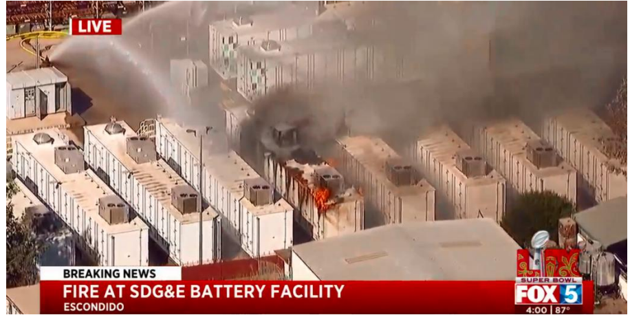
Escondido Substation BESS Fire – Media Coverage
