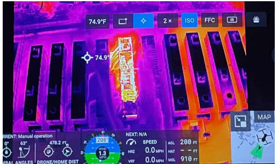
Escondido Substation BESS Fire – Thermal Image
