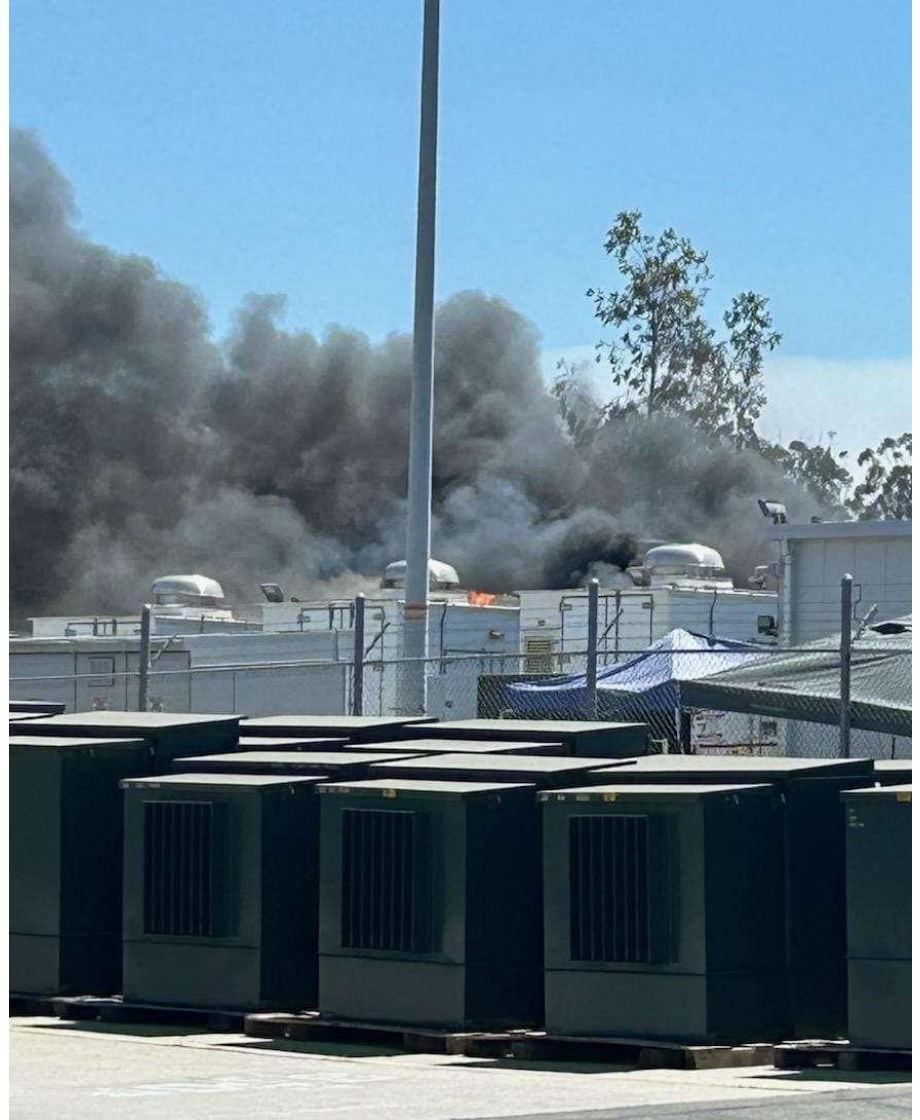
Escondido Substation BESS Fire – Particulate Plume
