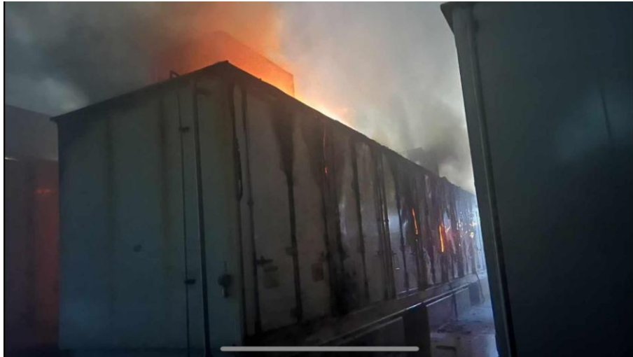
Escondido Substation BESS Fire – Involved Container
