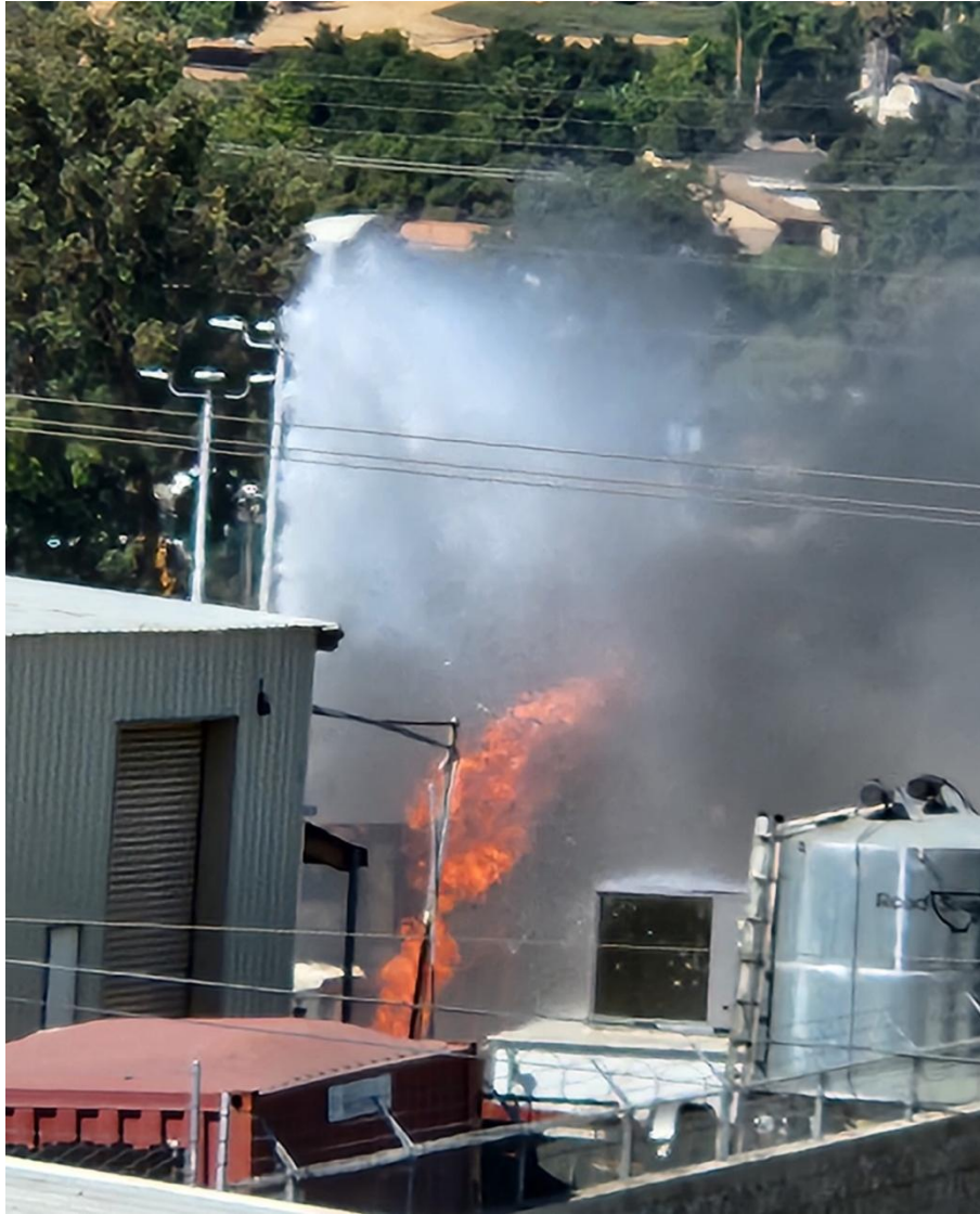
Escondido Substation BESS Fire – September 5, 2024
