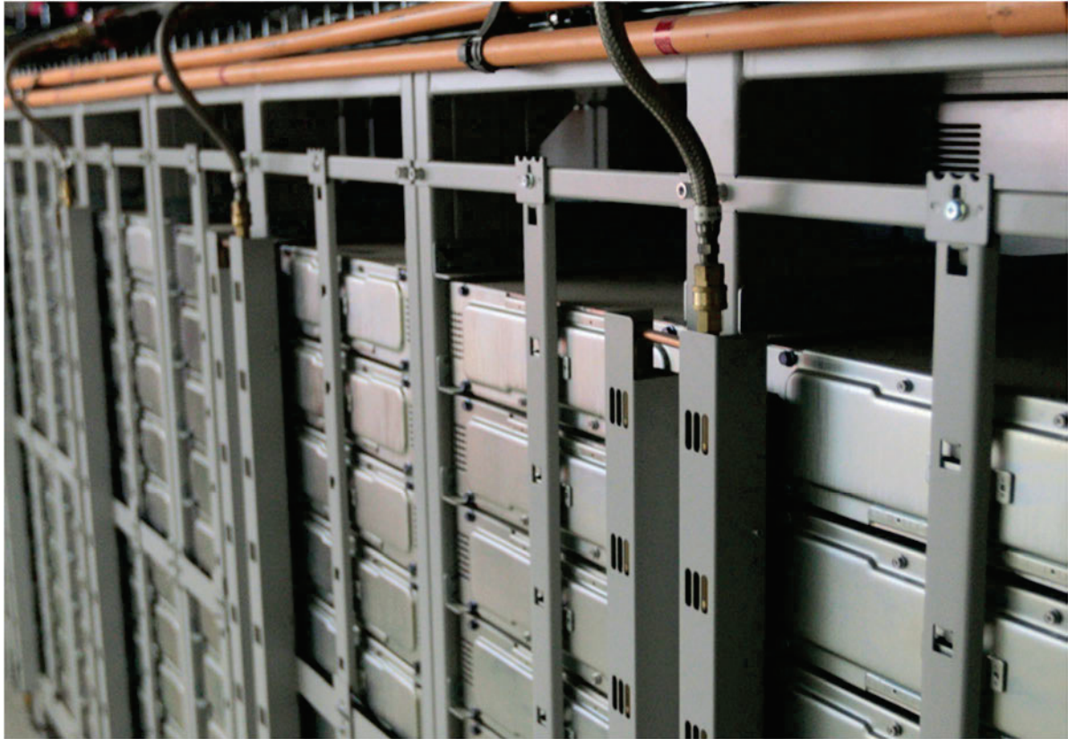
Figure 2: Backside of Indoor Battery Packs at Moss Landing BESS 3
