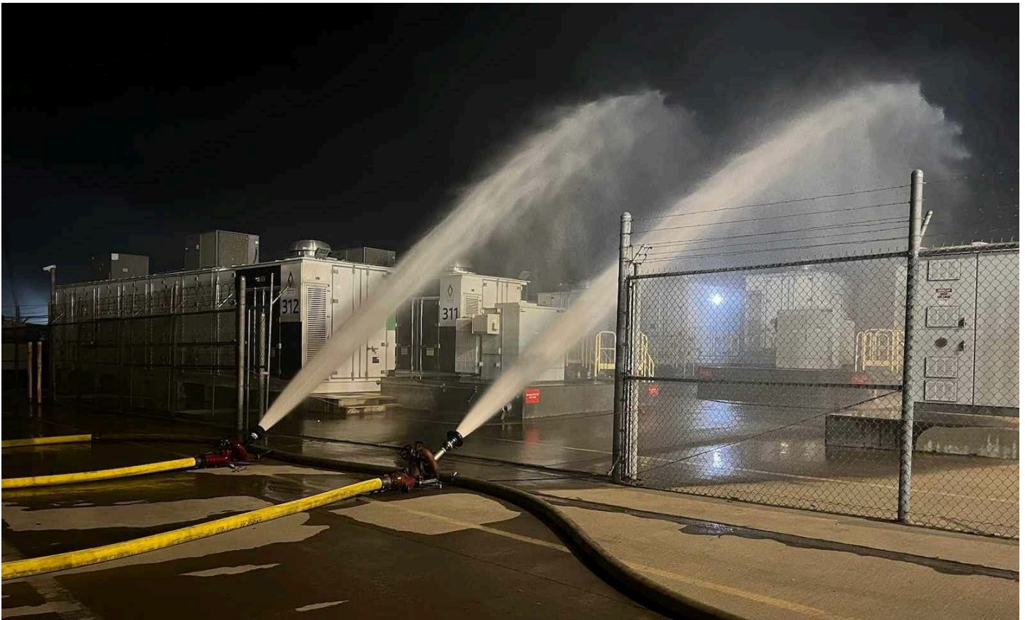
Escondido Substation BESS Fire – Propagation Suppression September 5, 2024
