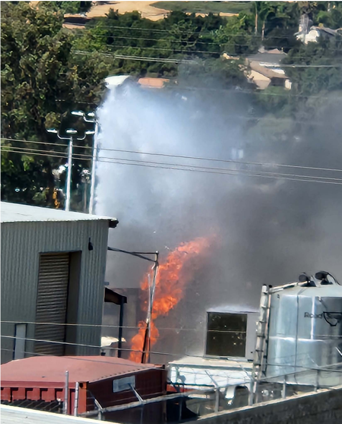
Escondido Substation BESS Fire September 5, 2024
