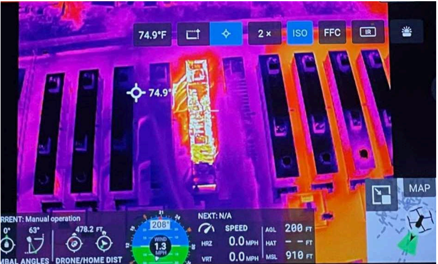
Escondido Substation BESS Fire – Thermal Image September 5, 2024
