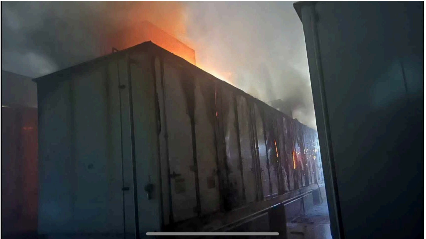
Escondido Substation BESS Fire – Involved Container September 5, 2024
