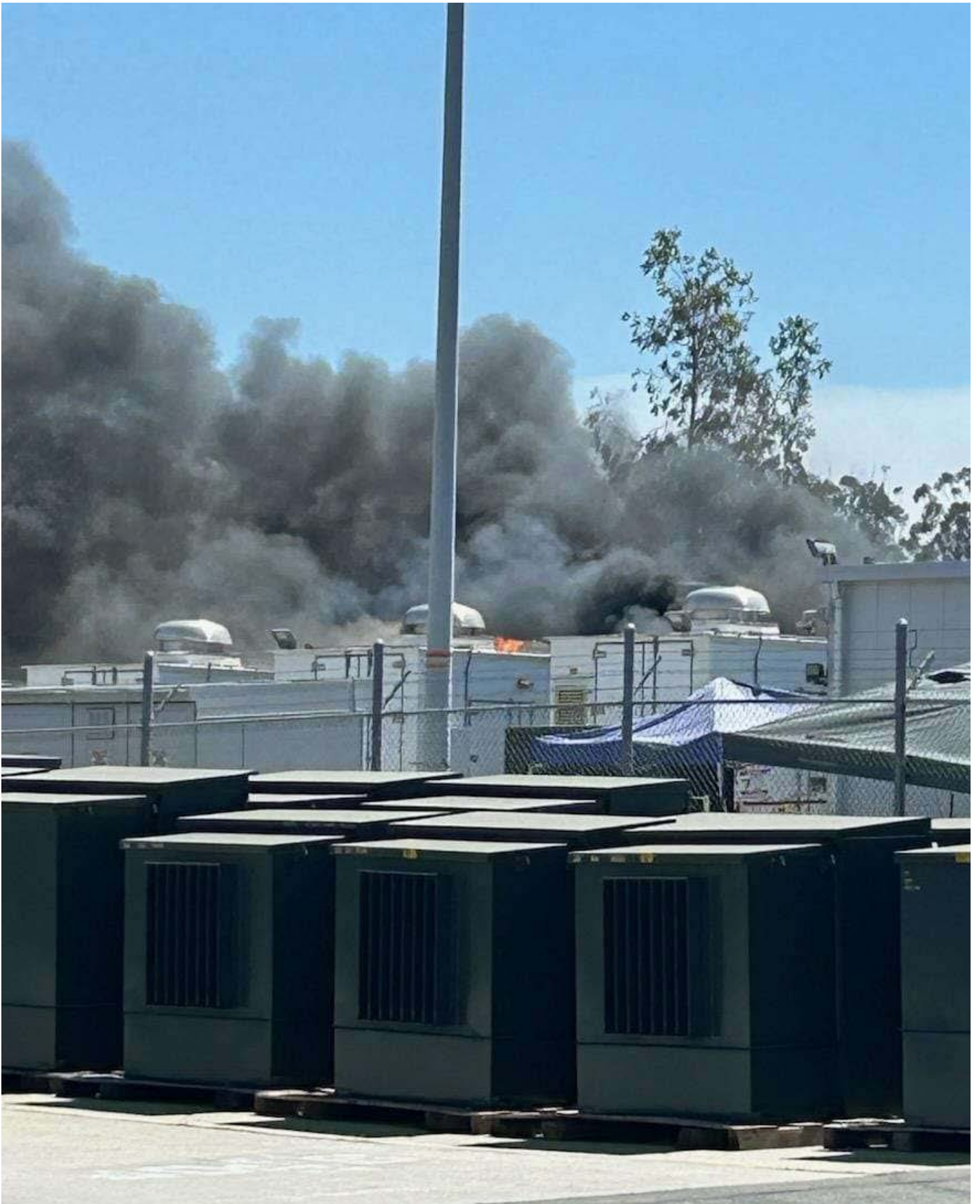
Escondido Substation BESS Fire – Particulate Plume September 5, 2024
