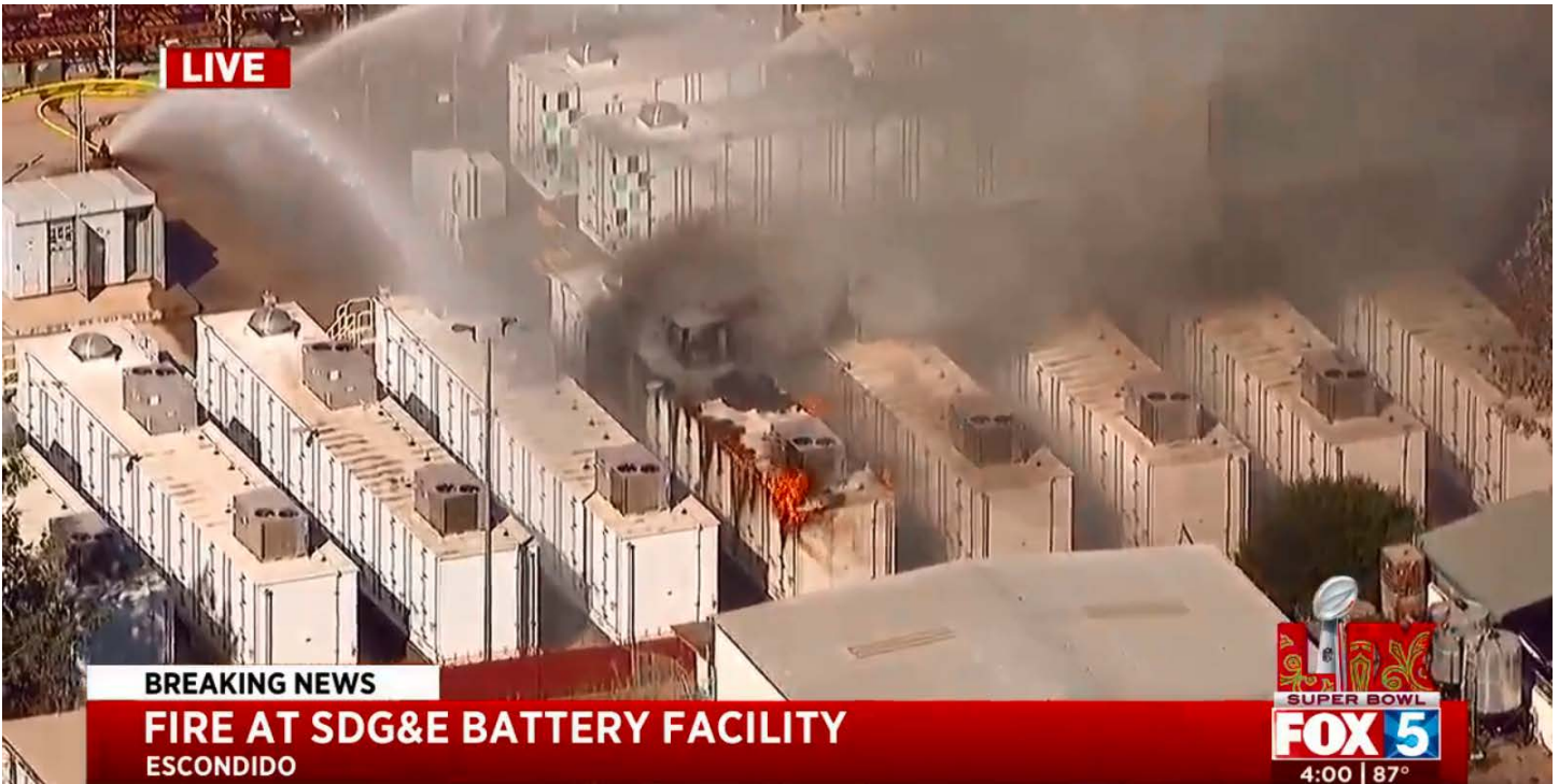
Escondido Substation BESS Fire – News Coverage September 5, 2024
