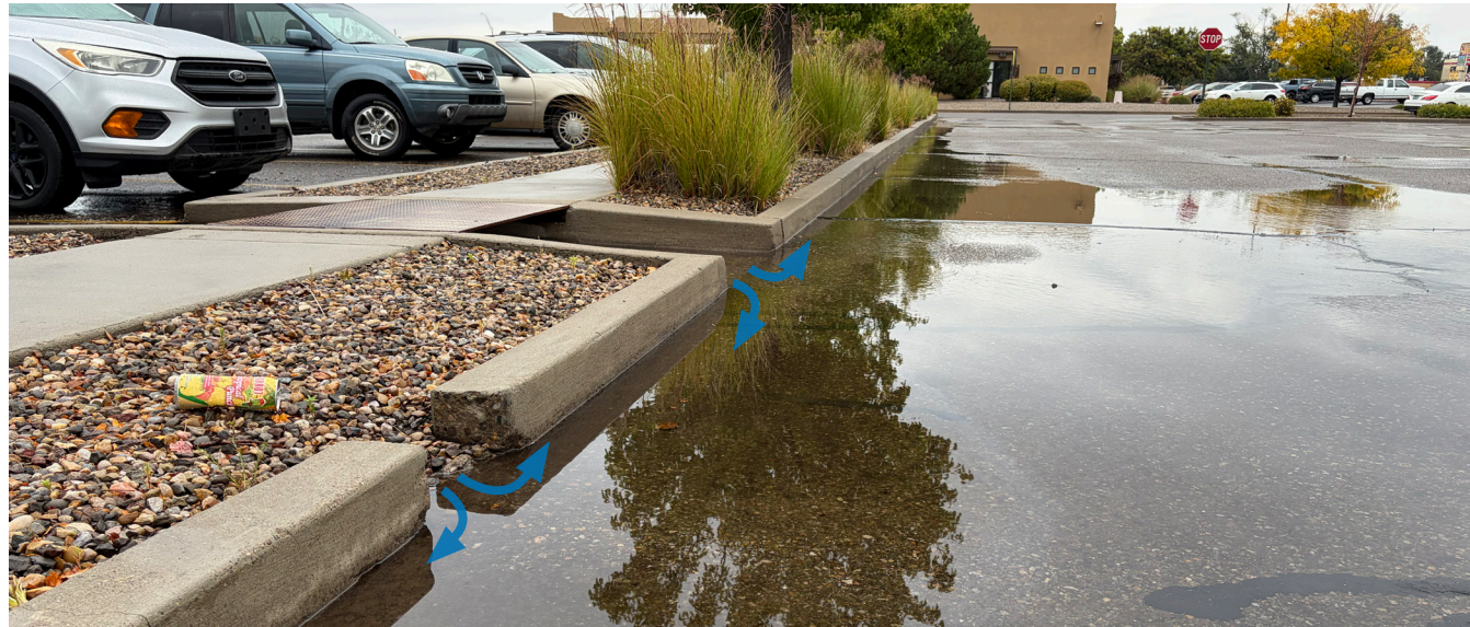
Standing water due to the absence of GSI in a parking lot.
