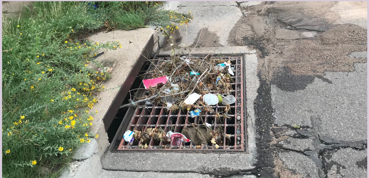
An example of trash carried by stormwater runoff collecting in a storm drain.
