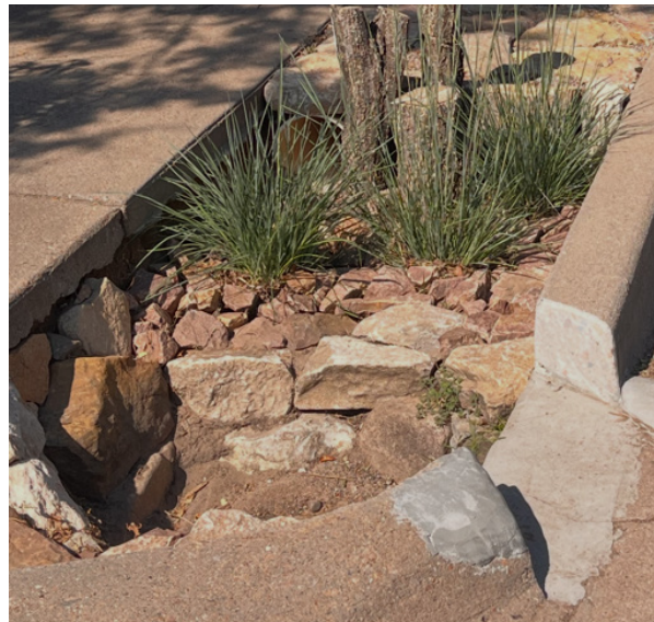
Sediment trap with float grass filter behind to block debris from entering the rest of the GSI feature, dry.
