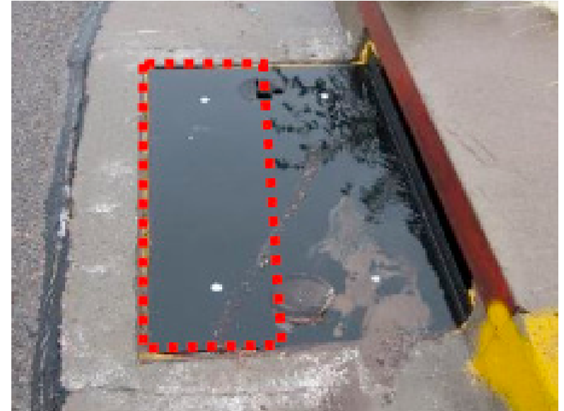
Drain cap showing how the omission of half its possible area (i.e. red dotted line) would redirect flow during smaller storm events, but drain larger runoff events.
