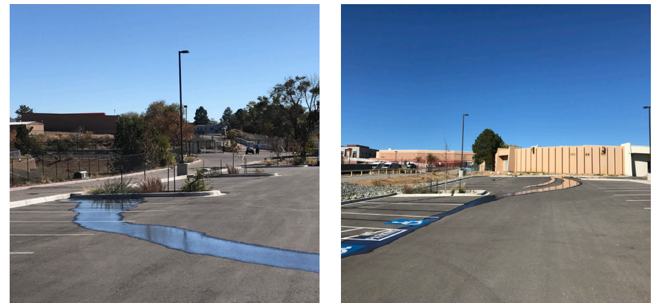
Figure 5. The rain garden on the left maximizes stormwater catchment because asphalt grades were installed properly. The rain garden on the right misses almost 2,000sqft of runoff (i.e. thousands of gallons annually) because asphalt grades were off by an inch!
