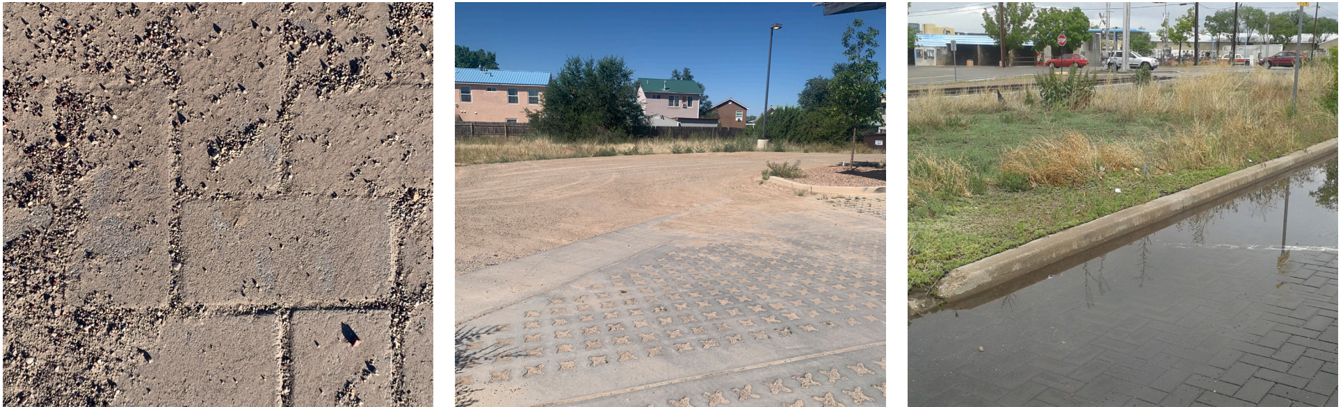
Figure 9. Examples of how unmaintained permeable pavers can lose infiltration capacity due to fine textures plugging the porous gaps (left and middle) which results in standing water on the surface (right).
