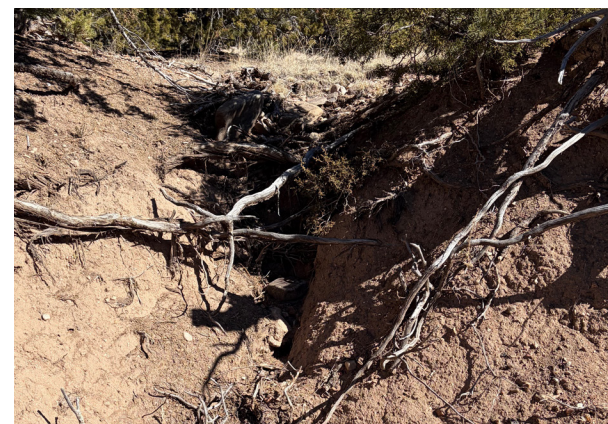
Exposed tree roots due to headcut erosion
