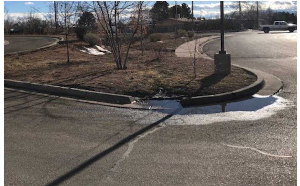
Neglected maintenance and absence of sediment trap result in soil build up that surpasses inlet elevation, blocking water from entering GSI feature.
