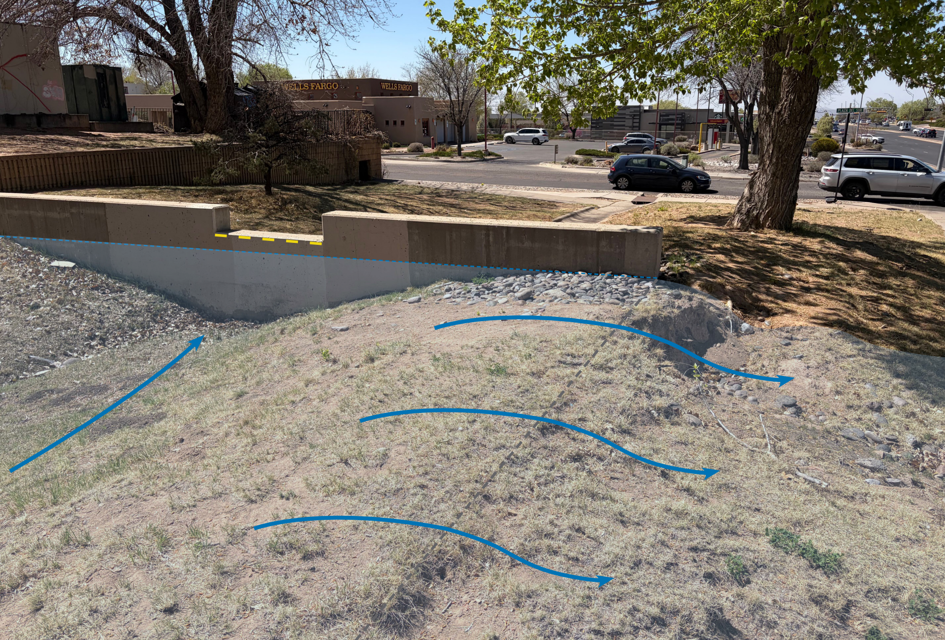
Figure 17. An example of basin edges (blue dotted line) that are lower than the intended pour over point on a weir (yellow dotted line) which leads to failure (i.e. blue arrows showing erosion from stormwater exceeding basin edge).
