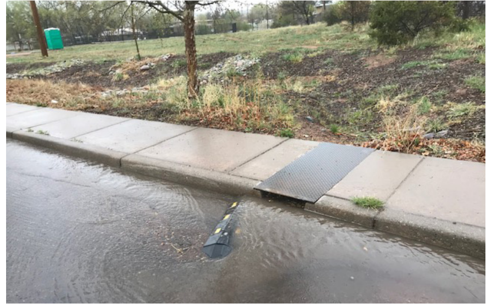
Consequence of sediment and debris build up: water cannot enter GSI feature.
