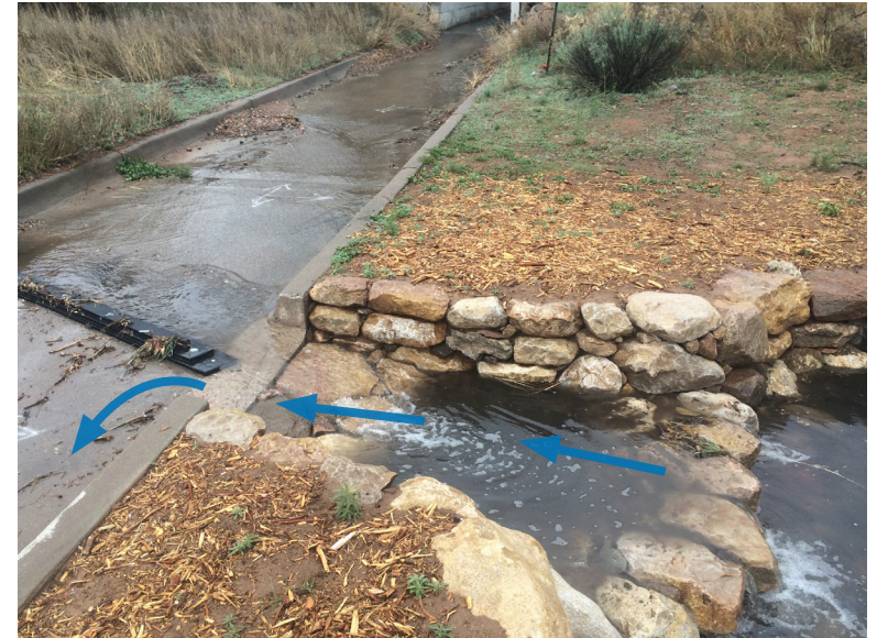
Curb cut can function as both the inlet and outlet when necessary.
