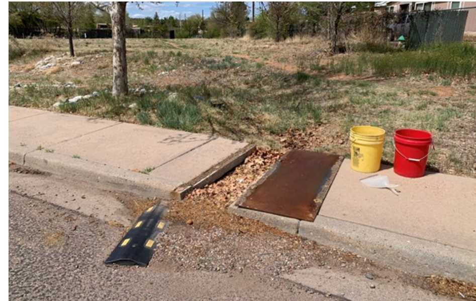
Sediment and debris built up at the inlet of a GSI feature due to lack of maintenance.
