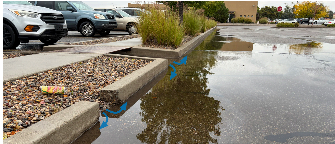
Standing water due to the absence of GSI in a parking lot.
