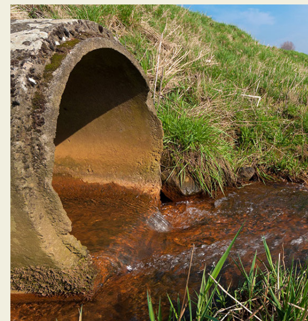
Unfiltered pollutants entering landscape from stormwater outlet.
