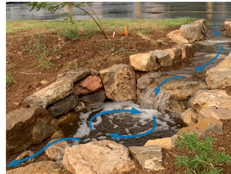
Zuni Bowl Slowing and Stepping Stormwater Down-Slope from Impervious Parking Lot Surface.
