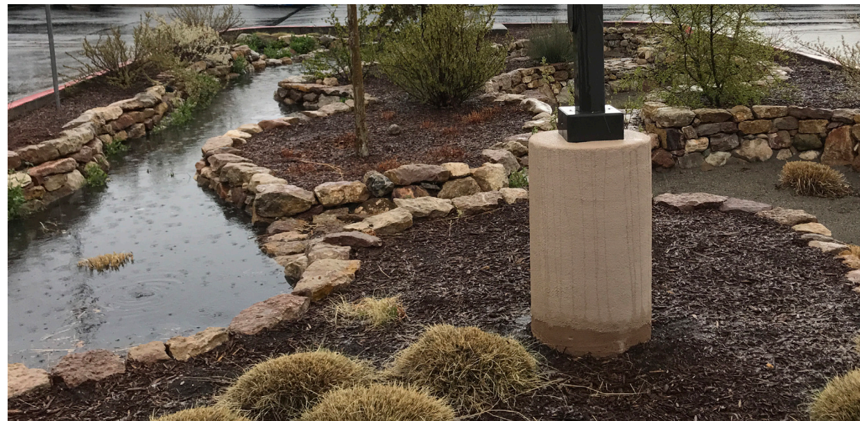
Figure 19. An example of a weir (blue arrows) in a rain garden which forces stormwater to pool a certain depth before it can overflow to the next basin. Weirs can concentrate stormwater near trees to enhance irrigation, above woodchip sponges to improve filtration, or simply to slow stormwater velocity as it passes through a GSI feature.
