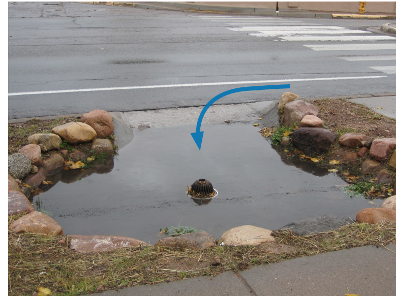
Wide Curb Cut Inlet with Armored Sides to Capture Flow Running Parallel to Opening.
