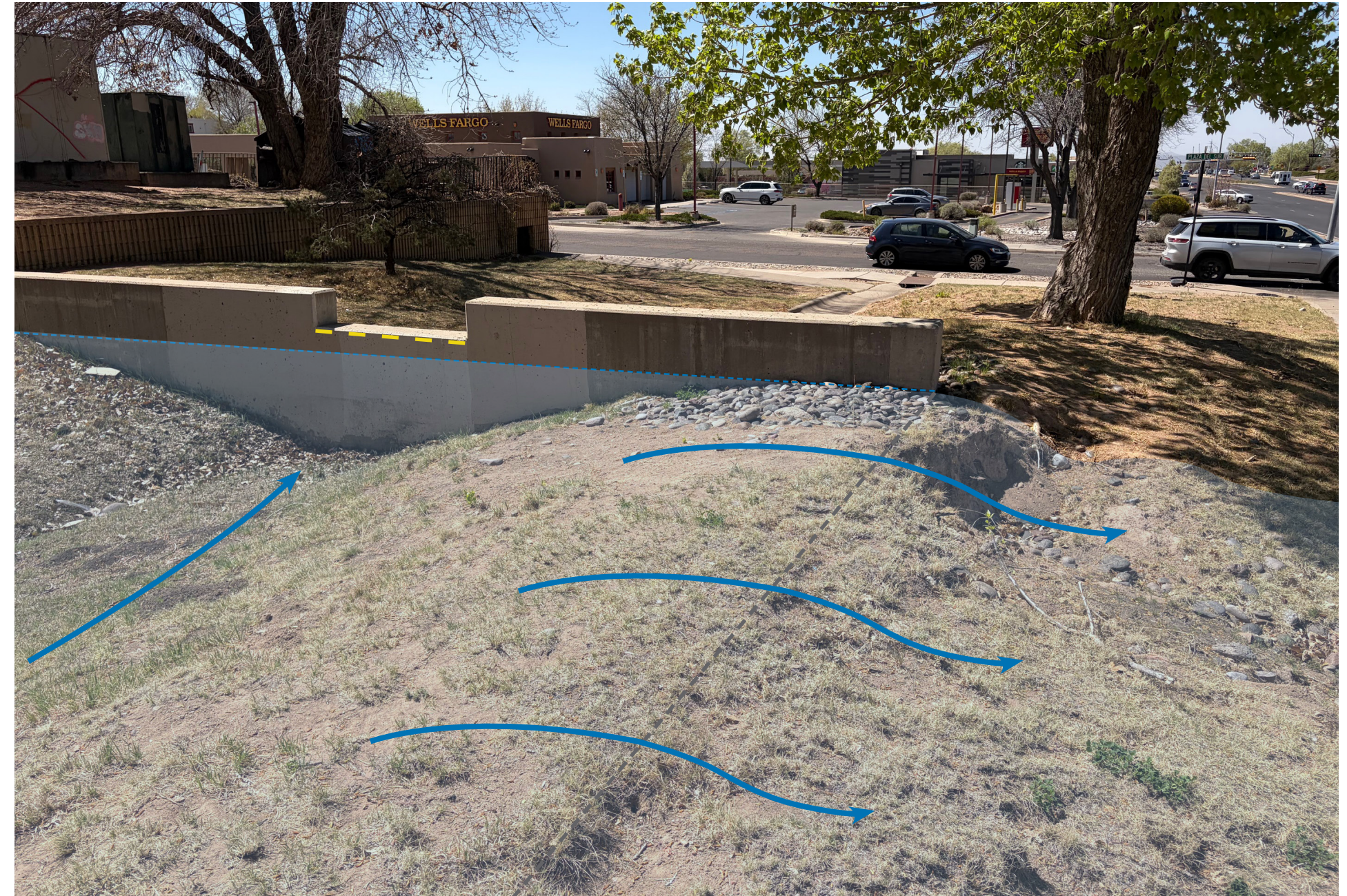
Figure 17. An example of basin edges (grey dotted line) that are lower than the intended pour over point on a weir (yellow dotted line) which leads to failure (i.e. blue arrows showing erosion from stormwater exceeding basin edge).
