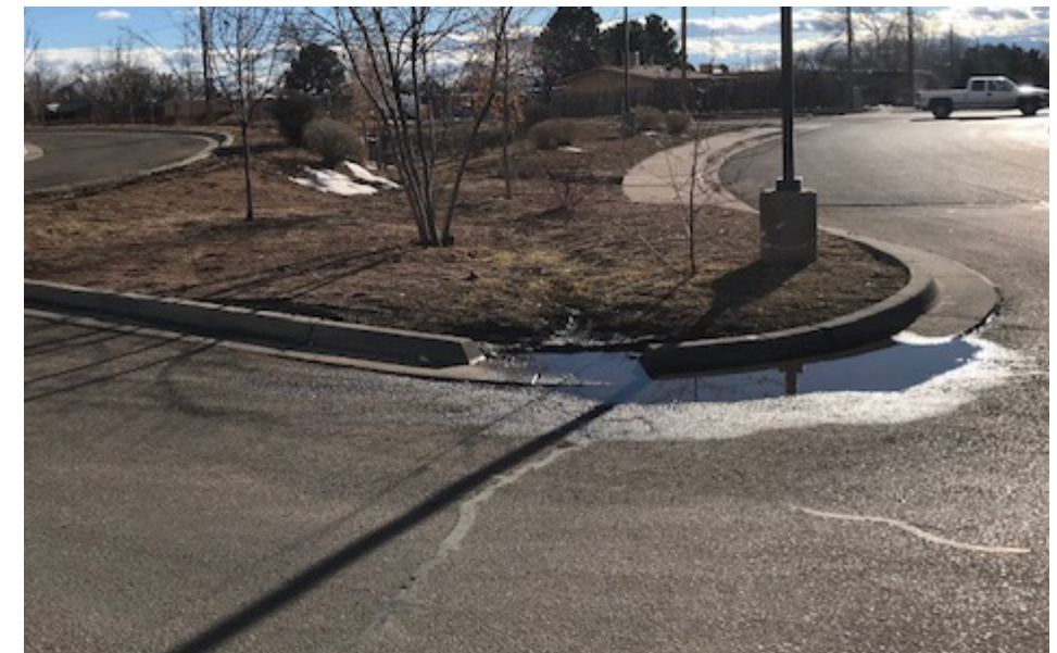
Neglected maintenance and absence of sediment trap result in soil build up that surpasses inlet elevation, blocking water from entering GSI feature.
