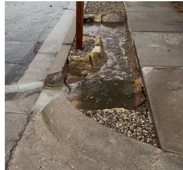
Water being directed into a sediment trap by a deflector and traveling through a rain garden feature. Note darker water in sediment trap, evident of its depth and collected debris.
