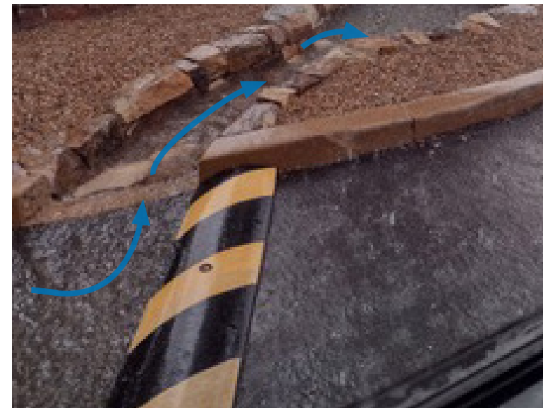
Speed Bump Deflector In Rain Directing Stormwater Runoff into Curbside Rain Garden.
