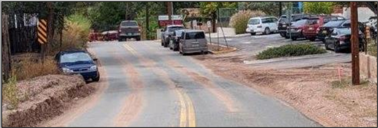
Figure 27: Sediment deposits on Bishops Lodge Road
