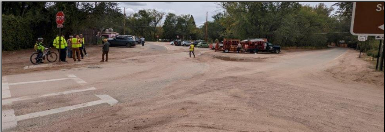
Figure 28: Sediment deposits on Arroyo Griego Road
