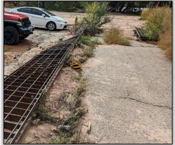
Figure 38: Decrepit infrastructure posing a safety challenge for pedestrians
